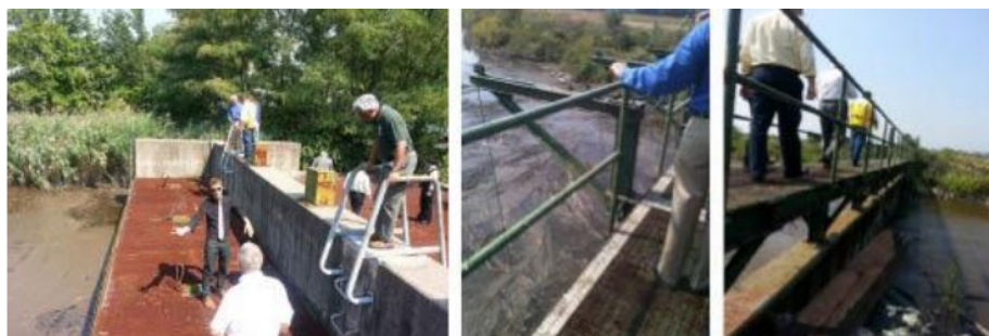
Figure 4-1: Physical Inspection of Existing Risk Reduction Infrastructure. Teams assigned by the New Jersey Department of Environmental Protection have endeavored to catalogue Superstorm Sandy’s impact on berms, tidal gates, and other existing risk-reduction infrastructure. Physical inspection is a key part of the State’s assessment of the current condition of measures to identify necessary repairs as well as opportunities to enhance existing measures to address future extreme weather events and maximize federal investment.
