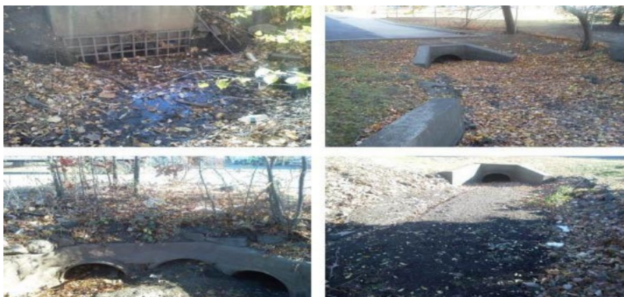
Figure 4-2: Drainage Systems, Moonachie/ Little Ferry. Addressing drainage issues could offer low-cost investment opportunities to increase New Jersey’s flood resilience. For example, bottlenecks in drainage systems, accumulated debris, and overgrowth may collectively exacerbate the impact of flooding and storm surge on communities. In addition, some drainage systems, constructed piecemeal over the last two centuries, have never been mapped. For example, Rutgers has been evaluating how minor drainage improvements can reduce flooding in the Moonachie/ Little Ferry region (pictured).
